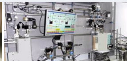
radon extraction rig
