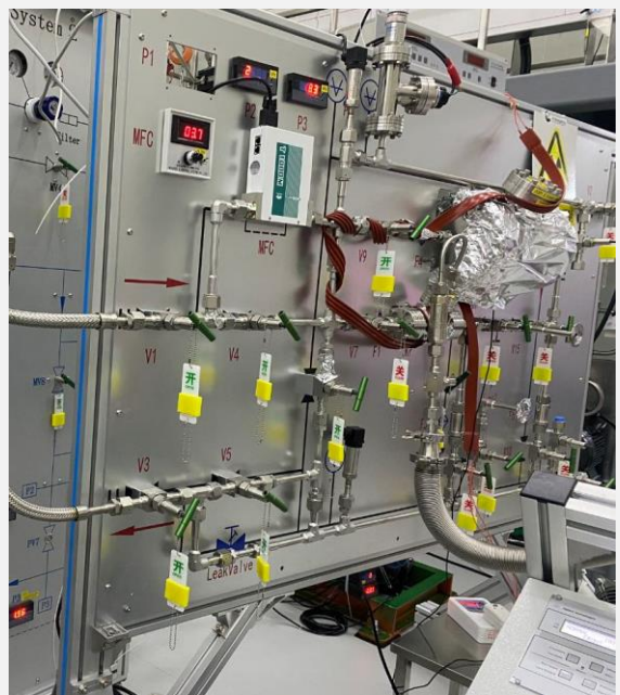
Gaseous source injection panel
